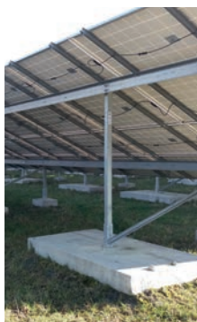
Photo 30: Fixed bi-pile table on concrete slab (© Idele)
