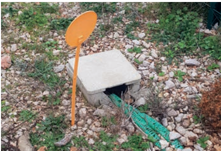
Photo 37: Example of a manhole that may be present in a photovoltaic park (© Idele)
