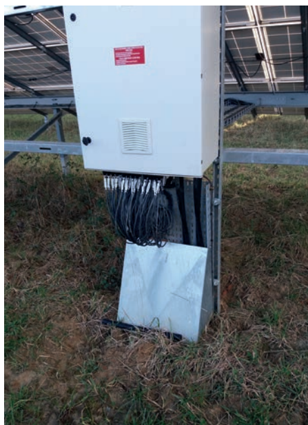
Photo 33: Electrical wiring left visible at low height that can be gnawed by animals (© Idele)
