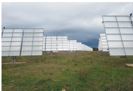
Photo 16: 2-axis tracker photovoltaic panels in Grabels (34) (© Idele, park managed by Neoen)
