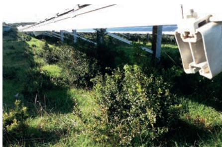
Photo 27: Invasive bushes not consumed by the ewes, ultimately harmful to the performance of the park (© Idele)
