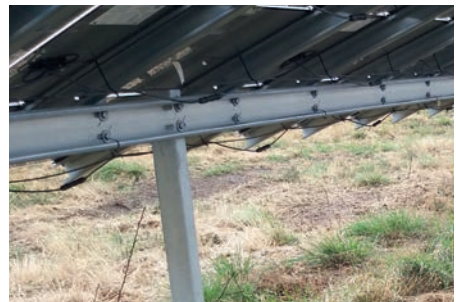
Photo 38: Example of fixing electric cables with cable ties at the back of a photovoltaic panel (© Idele)
