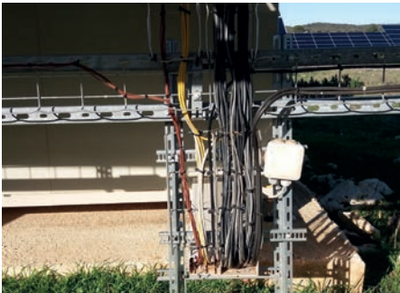
Photo 36: Wiring left visible (© Idele)
