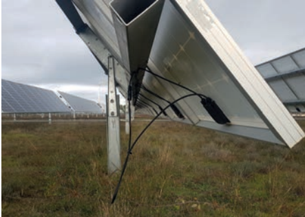
Photos 34 and 35: Electric cables tend to hang low behind panels, creating a risk of strangulation, especially in young animals. (© Idele)
